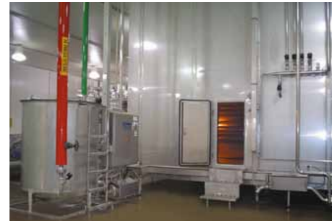
Recirculating Clean-In-Place (CIP) system
